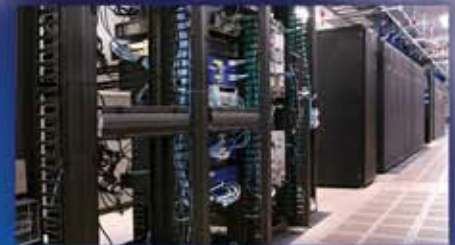
We Specialize in Data Center Cleaning
